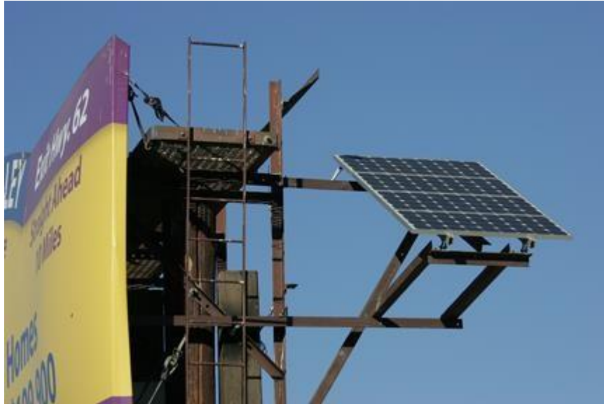
Figure-1: Solar powered light for Hoarding
