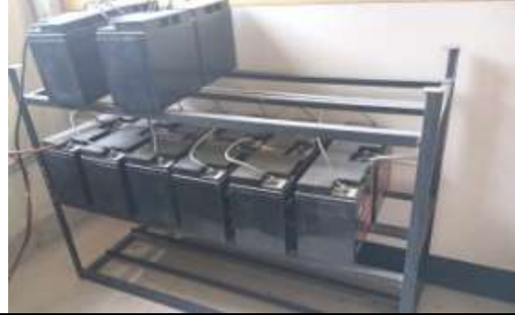
Power Inverter Batters
