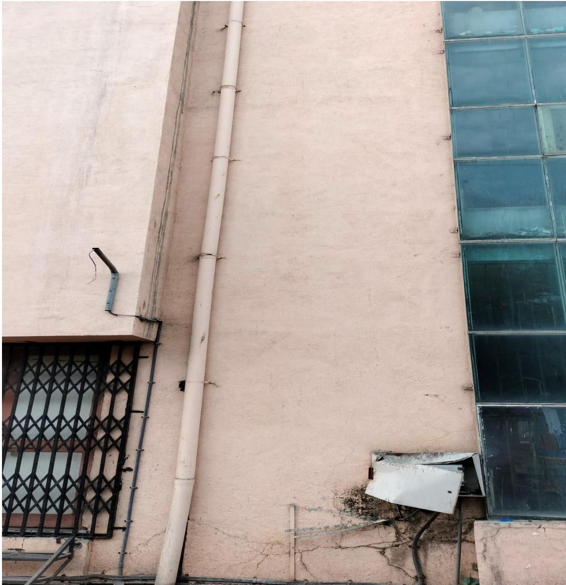
Photo-4: View of rain water collection from building
